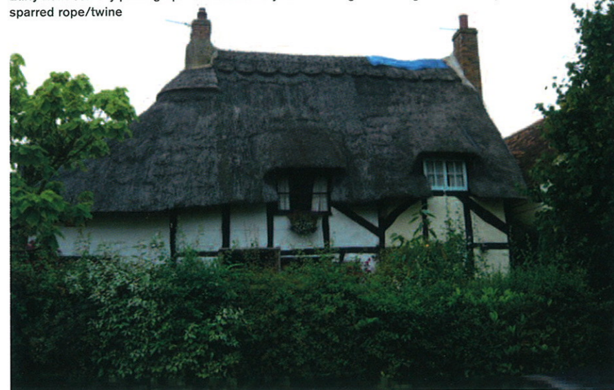
One hundred years later, 'modernised' with raised block-cut patterned ridges, held by decorative liggers, and new wallhead dormer windows. Right side now finished with wheat reed, left with water reed, variously repaired, all under galvanised steel netting
