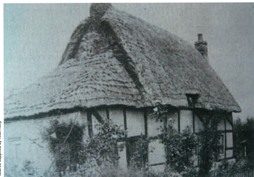
Early 20th century photograph of 17th century listed cottage with long straw thatch, fixed with sparred rope/twine
