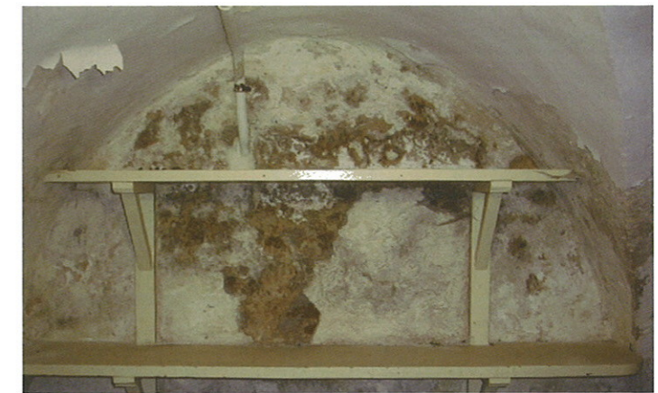
Figure 3 – Spalling and delamination of plasterwork, caused by masonry salts
