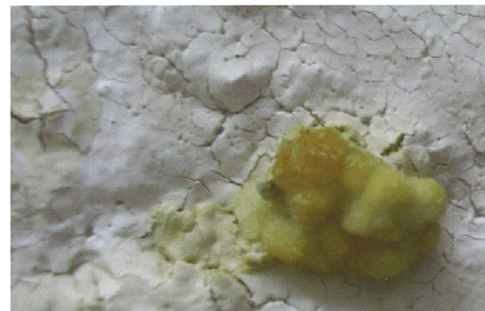
Figure 2 – The staining and flaking of historic paint finishes with surface fungal growth
