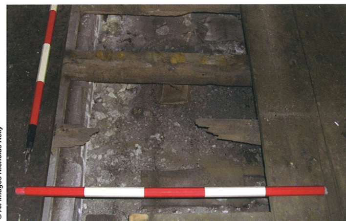
Figure 1 – The decay of timbers caused by repeated saturation (note the salt efflorescence to sub-floor brickwork)
