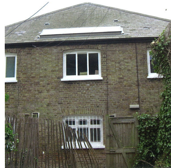
Solar water pre-heating panels, sympathetically installed to reflect industrial rooflights
