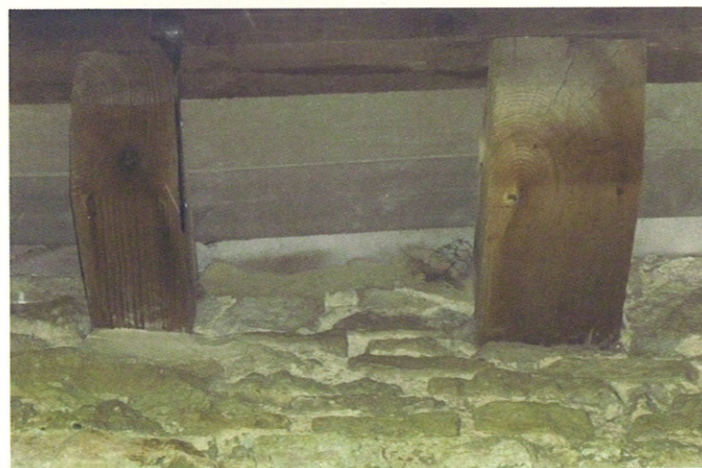
Image 2 – An illegal partial obstruction of a roost entrance following building works. The fur-oil stain to the soffit board indicates a bat roost entry point, obstructed by recently applied mortar
